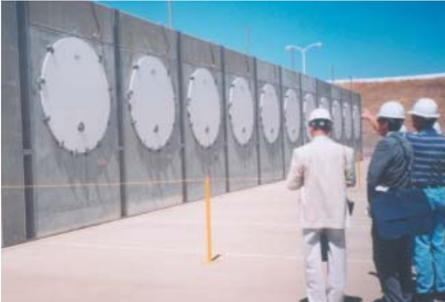
▲ Spent nuclear fuel dry storage in modules
